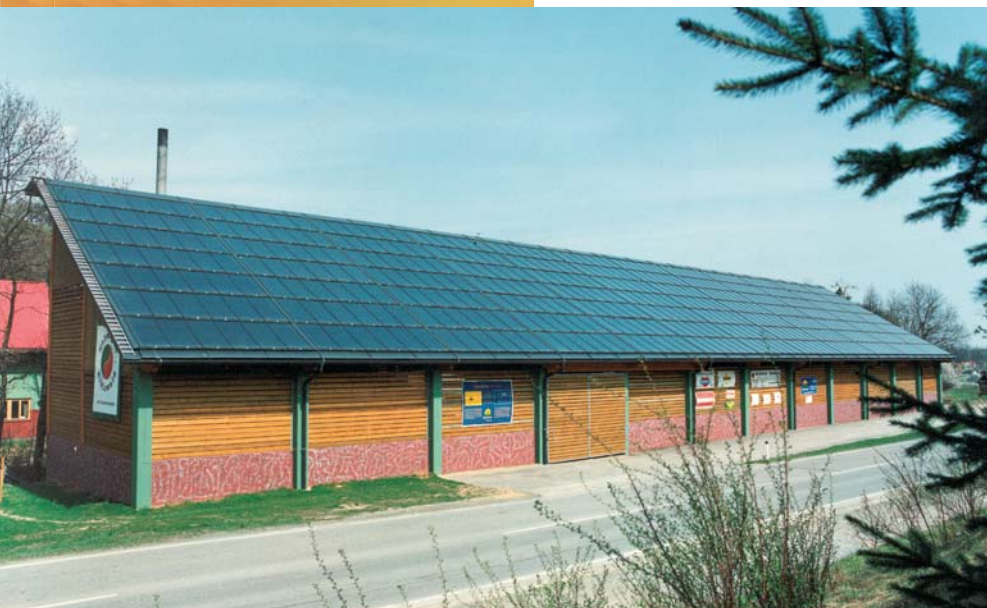
Collector area at storage building
