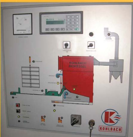
control center St. Oswald
